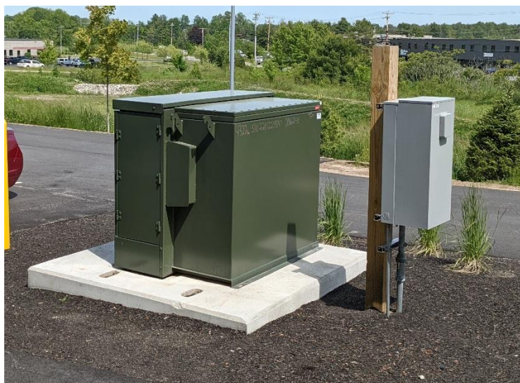
Figure 7 1 Ledgeview Drive Electrical Distribution Transformer
